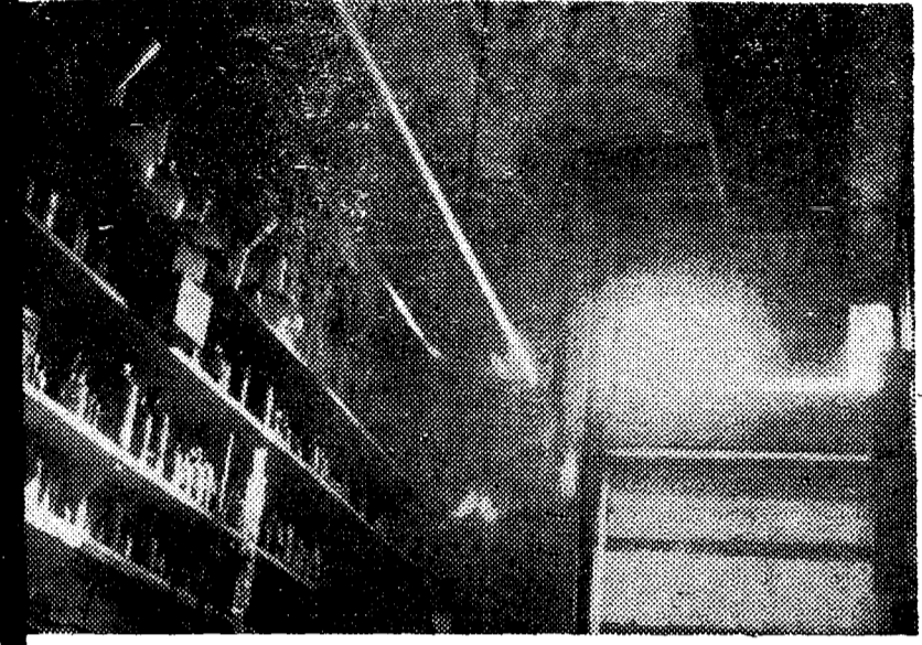
FALLING PLASTER from ceiling of research laboratory endangers chemists.
