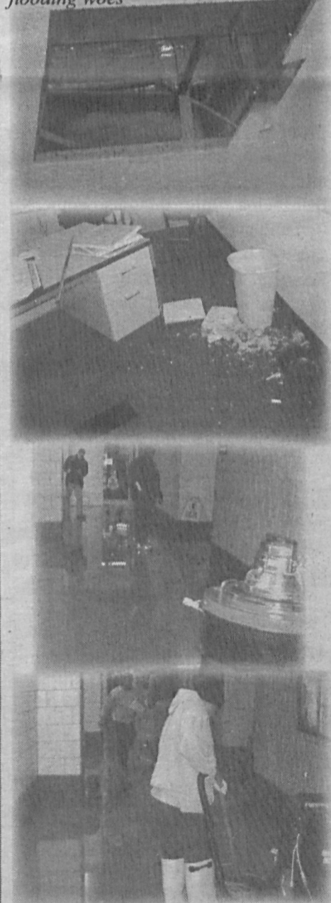
These four shows the horrible conditions of the school and its flooding woes
